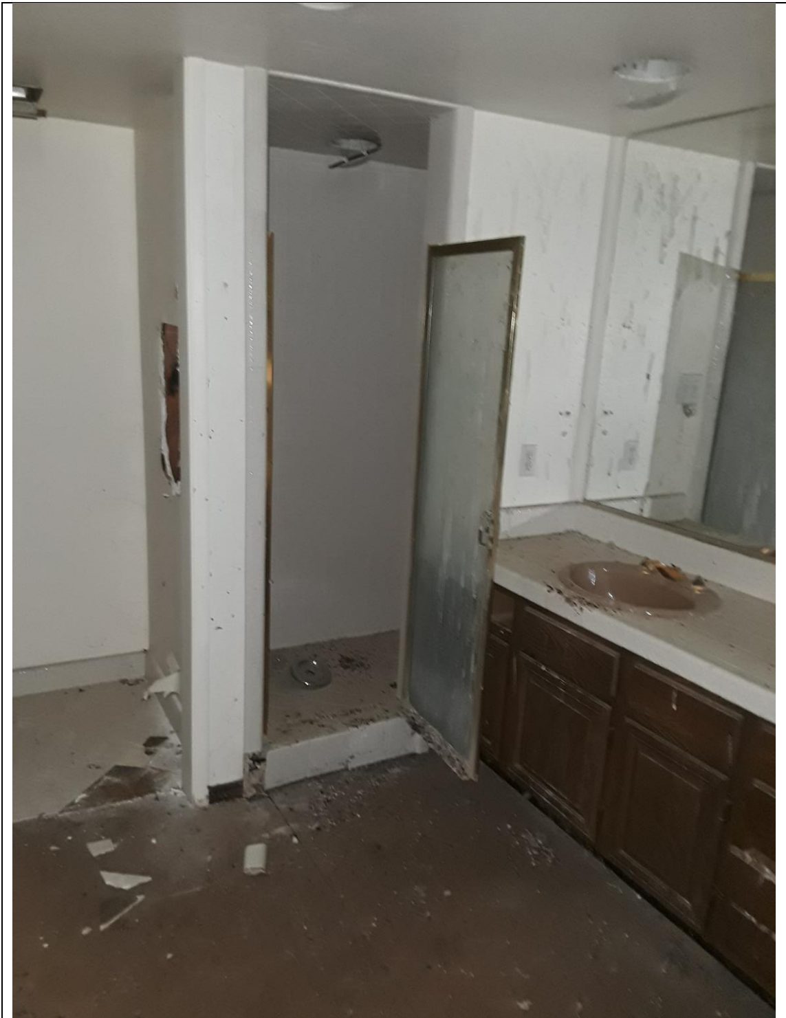
Photograph #3: Lead containing white tile (glaze) in shower/bathroom (LBP).
