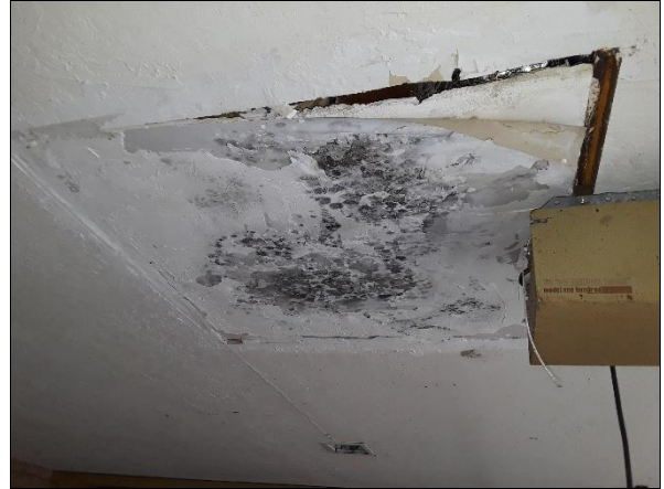
10. Moldy Drywall In Garage Tested <1% (Trace) For Asbestos Fibers
